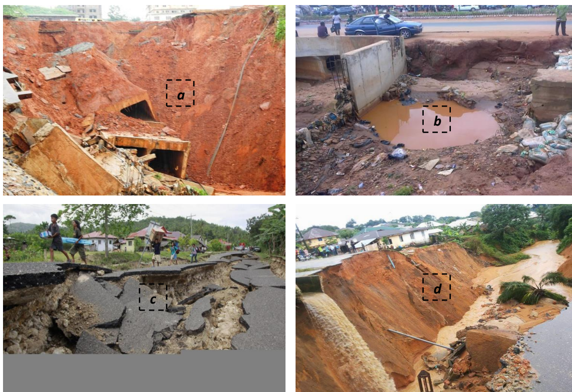
Figure 2 The impacts of erosion on: (a) urban drainage infrastructure and underground utility, (b) ongoing urban development project, (c) road network, and (d) causing land degradation.
